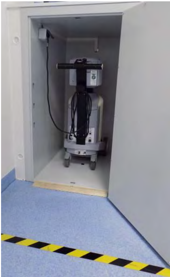
Fig. 2: Safe for secure storage of afterloader in accordance with DIN 25422
